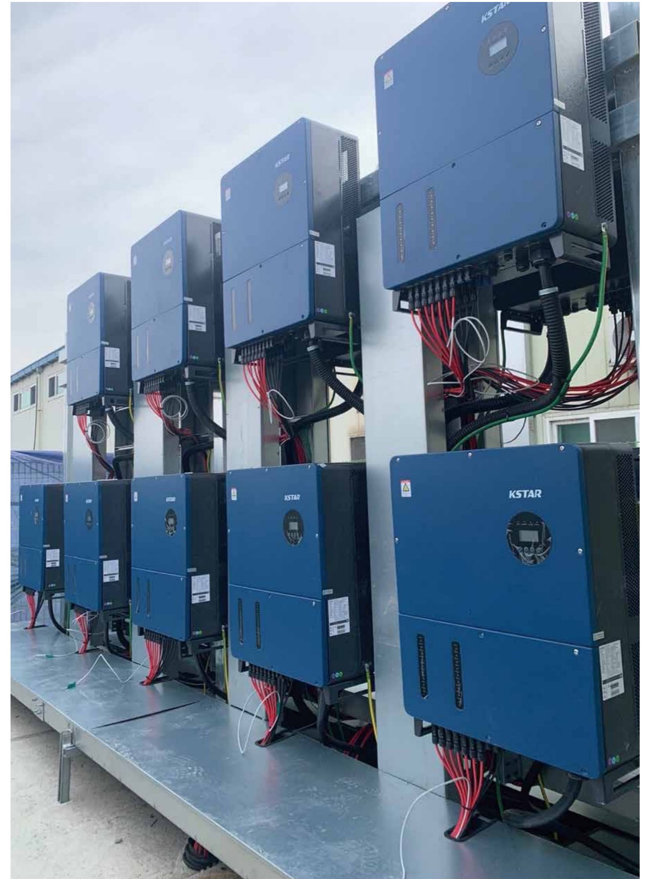
11 C&I Project in Daejeon 1MW, KSG-60K-A
