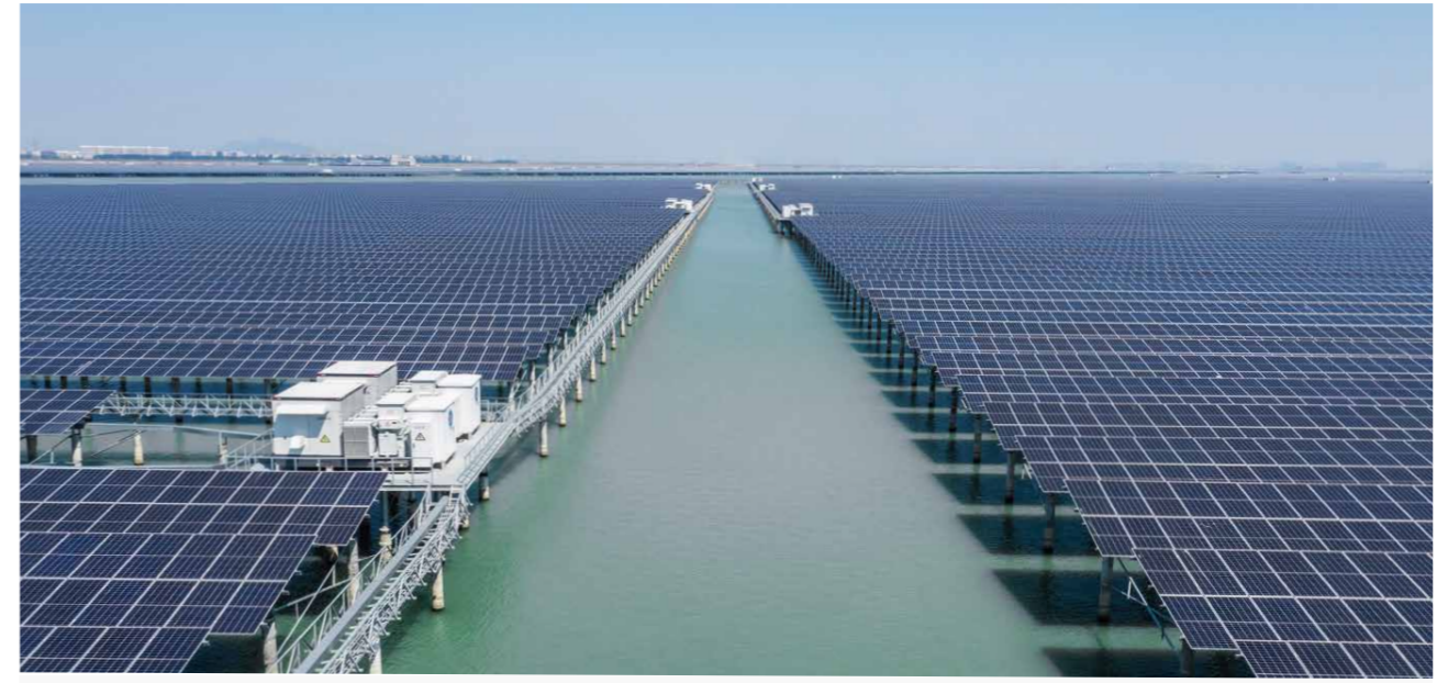
06 Utility Project in the Zhejiang 550MW Watersurface PV Plant
